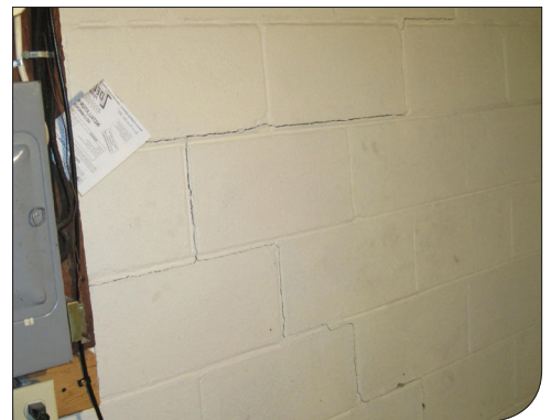
Stair stepping cracks in concrete block
